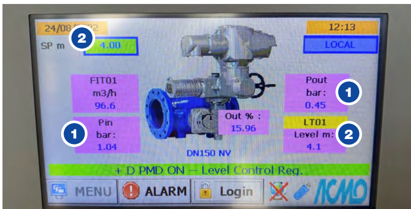
Key for the screen above: (picture shows reservoir level high - valve closing)
