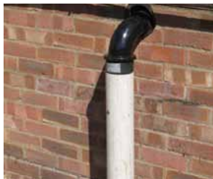
Gas taken into the building
